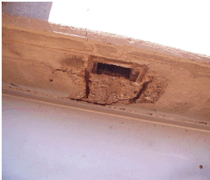
Figure 9-2. Corrosion Damage due to Concentrated De-icing Solution at Drain Site.
