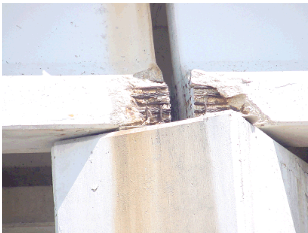
Figure 9-5. Chemical Solution Corrosion Induced Beam Damage Created by Failed Joint and Poor Concrete Cover over Beam Ends.
