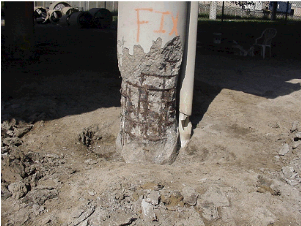
Figure 9-12. Damage Created due to the Salt Storage.
