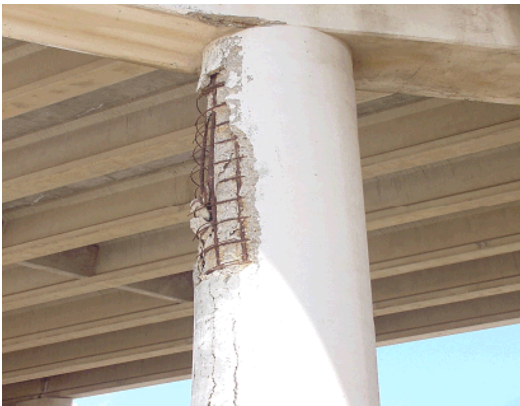
Figure 9-9. Column Deterioration from Chemical Solution Contamination.
